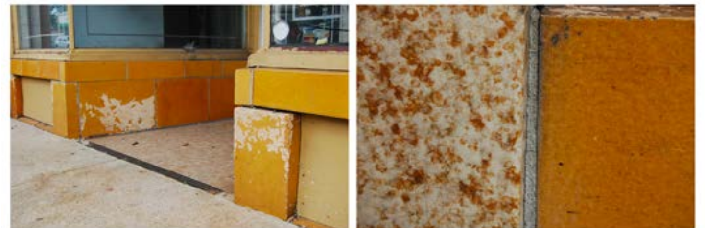
Superficial defects occurring along the base. On the right, a detail of two glazes on the building.
